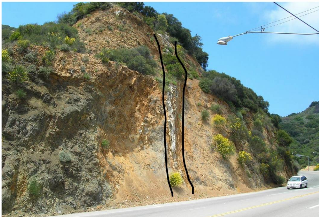
FIGURE 22. Site F, A view of a previously unmapped fault, which was identified during this study but does not correlate with any the study's current seismo-lineaments. Note vehicle for scale.
