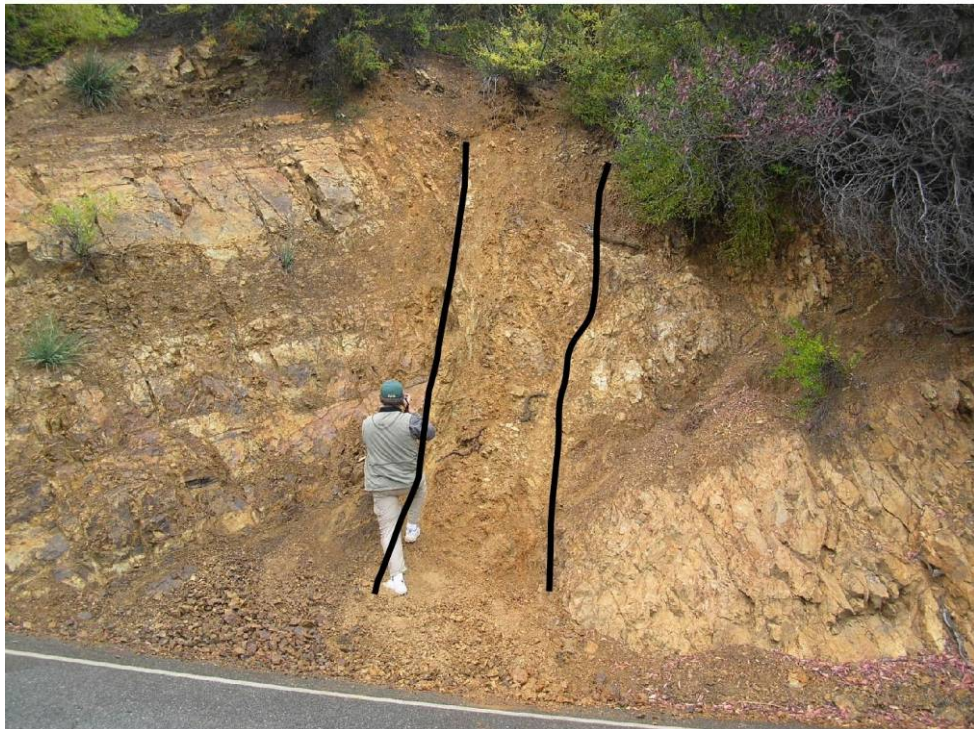
FIGURE 20. Fault at site D, an uninterpreted photograph at top. The same photo below with fault interpretation. Black lines indicate the edge of the fault zone.
