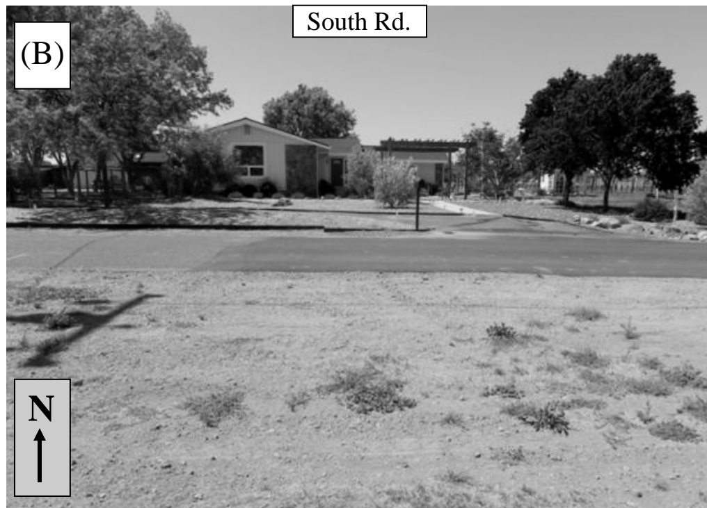
Figure 11. Examples of earthquake damage repaired in the Napa area. (A) Crack across South Road as observed immediately after the South Napa earthquake in August 2014, modified from Morelan et al. (2015). (B) Viewing the area from the opposite side of the road, it is evident that the damaged section of road has been patched. Patching is characteristic of many repairs in the Napa area, and was helpful in identifying areas in the field where rupture could have been seen immediately after the earthquake.
